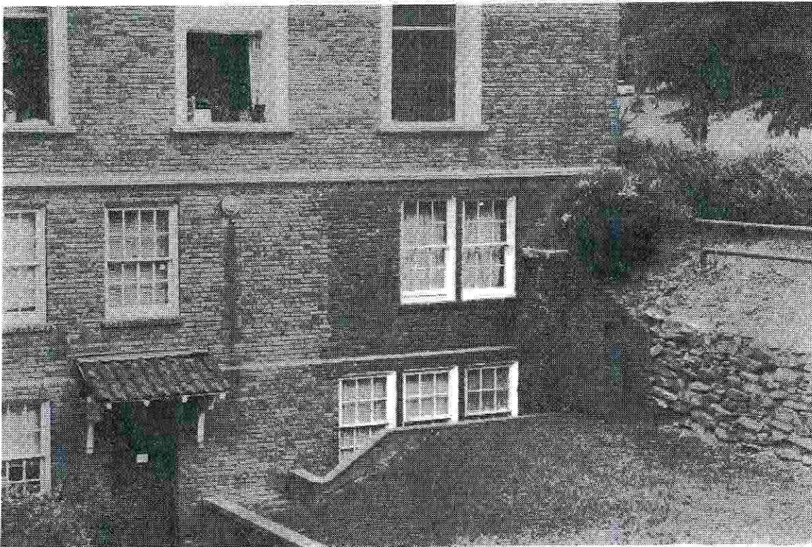
Figure 5: Non-matching brickwork at the YMCA detracts from the appearance of the south facade of the building.
